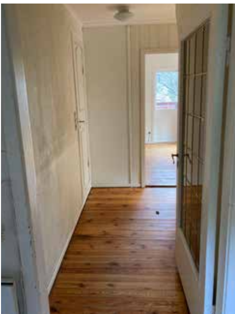
Gang inn mot stove 2
